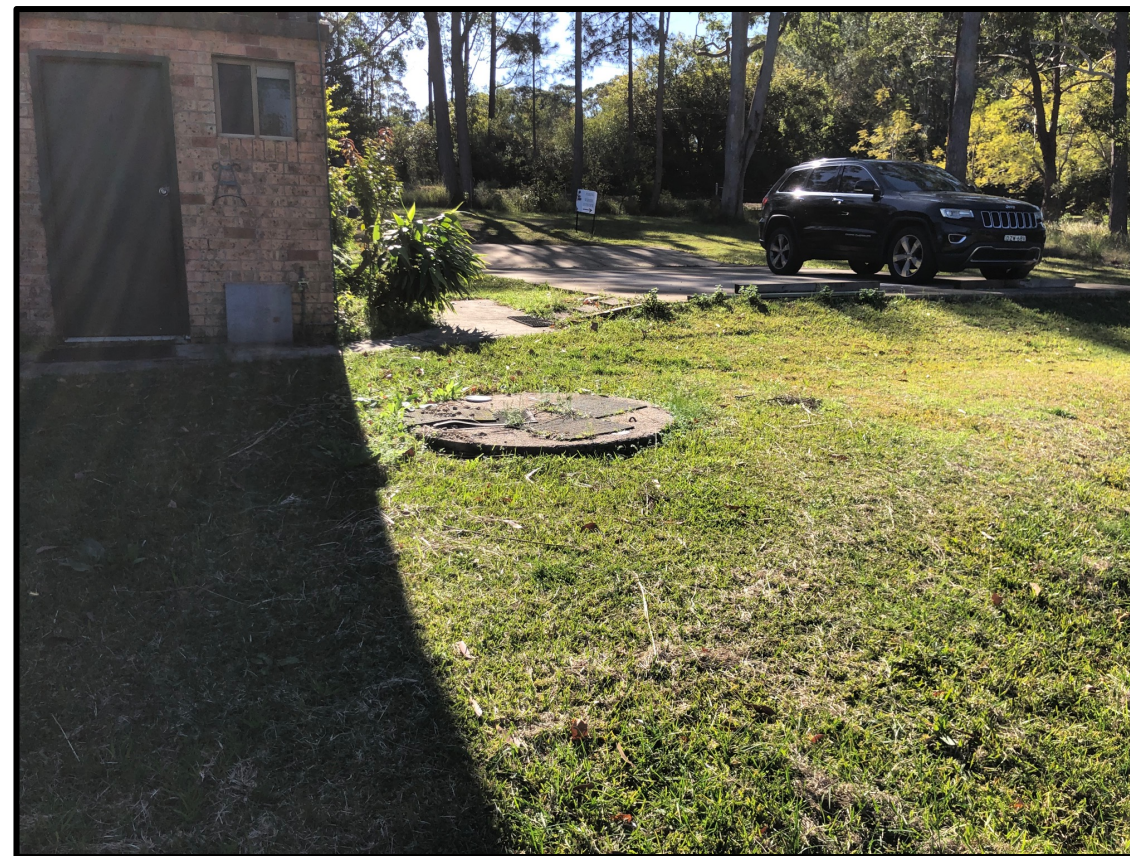
Figure 24. Septic tank at no. 54 Ferodale Road.
